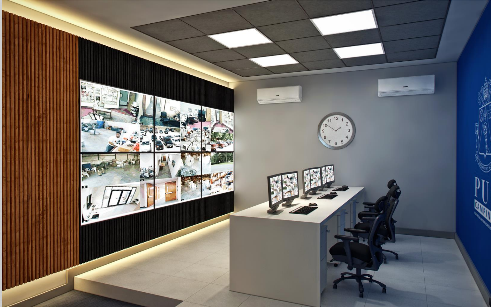
Puc Campinas Monitoring Room – Campinas/SP.
